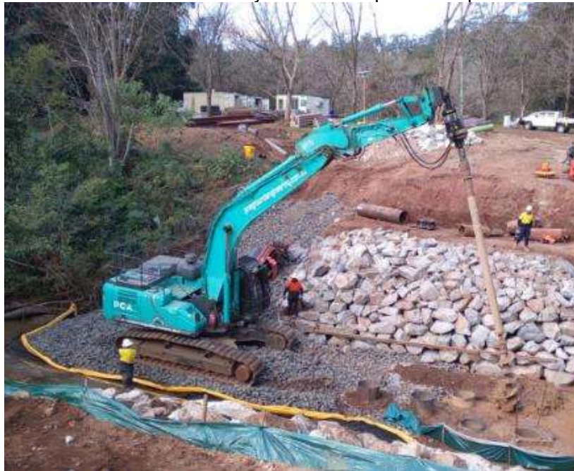
Excavator mounted pendulum pile boring rig with extendable Kelly bar and access ramps –
