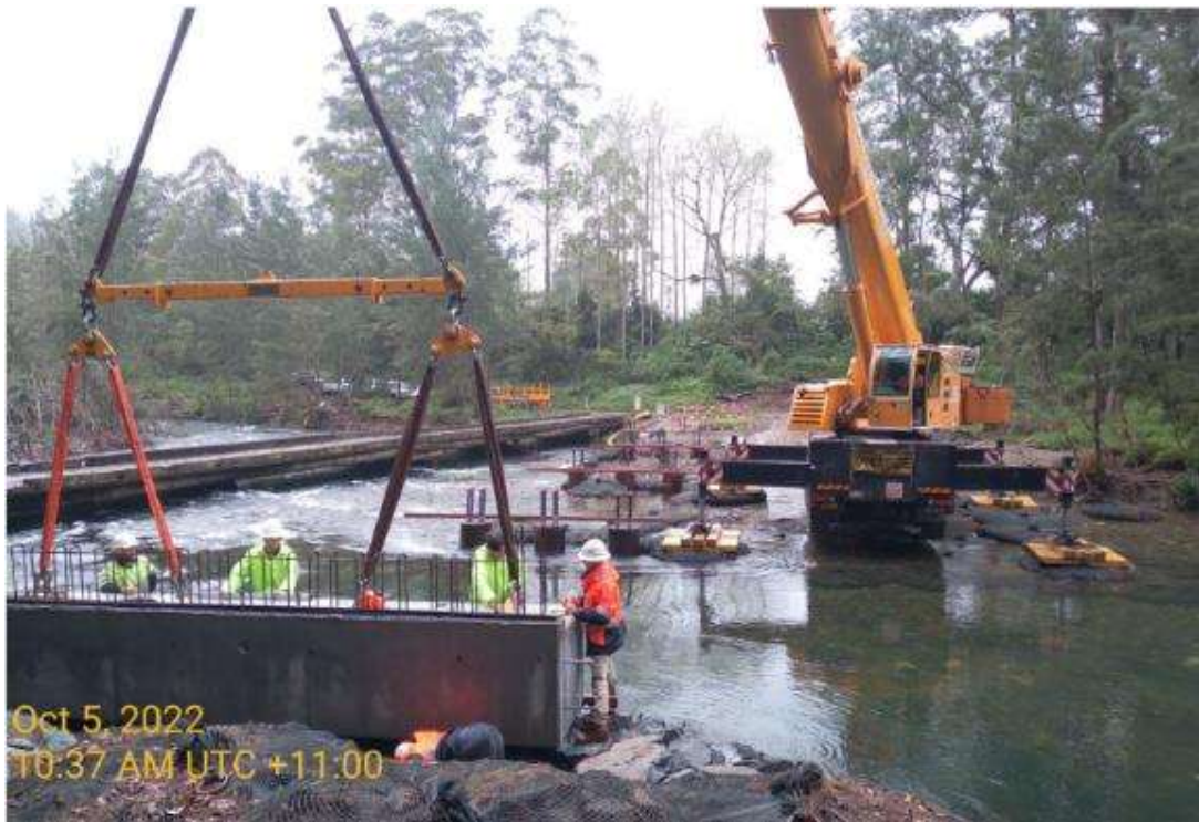
Rock bags used as an access track and crane platform for landing precast components
