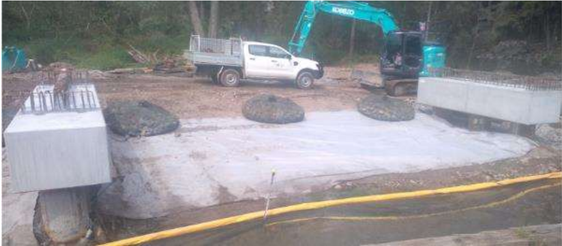
Rock bags used to pin down geofabric with boom adjacent in water
