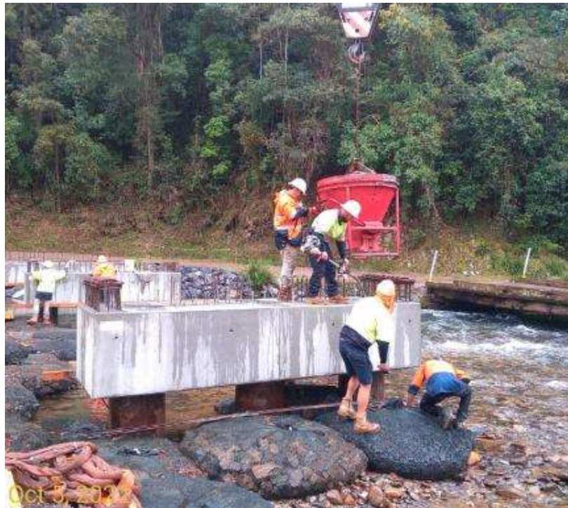
Kibble being used for on-site pours at headstocks near water to control concrete
