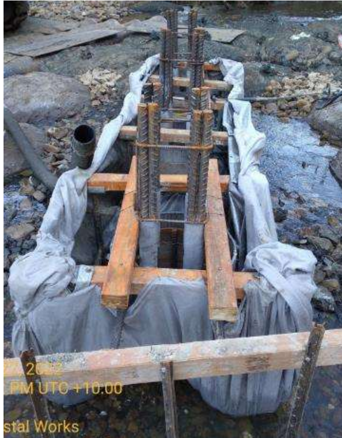
Containment system used for pouring concrete bored piles to prevent concrete overpour entering the waterway
