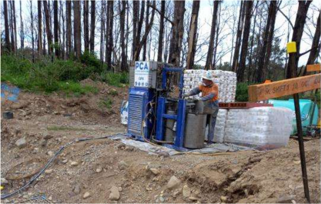
On-site grout mixing station for rock anchors up on banks away from anchors
