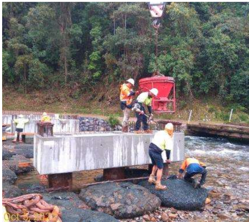
Kibble being used for on-site pours at headstocks near water to control concrete
