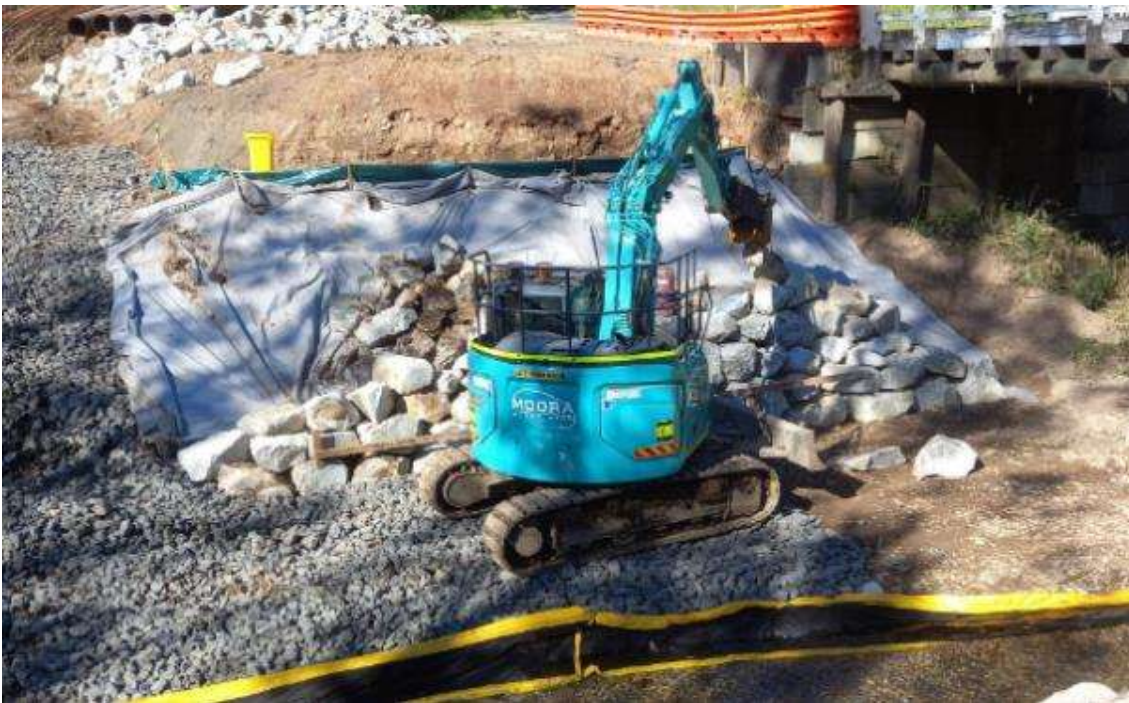
Riverbank access ramp and working area and rock scour protection with excavator
