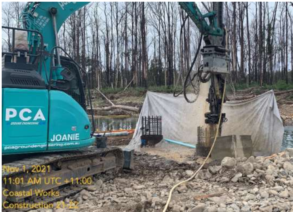
Excavator mounted rock anchor drilling setup (7-12t sized machine) with splatter screens used next to waterway
