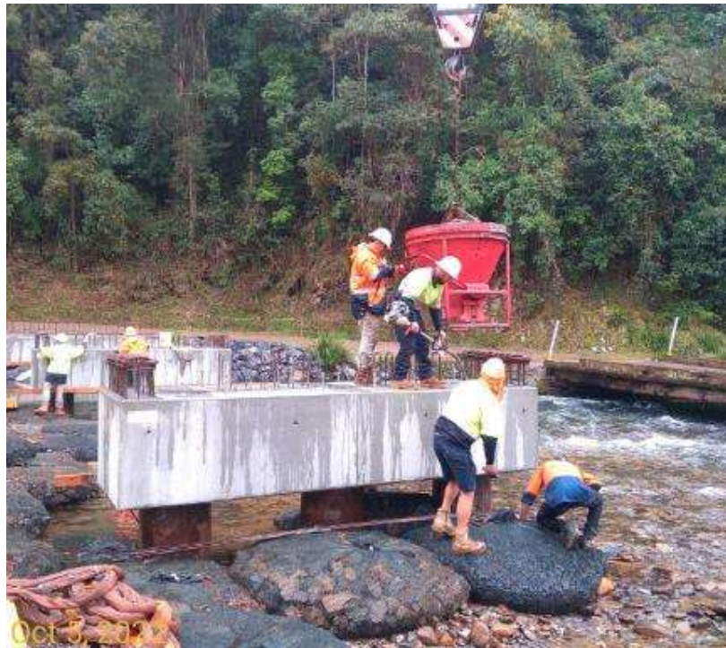
Kibble being used for on-site pours at headstocks near water to control concrete
