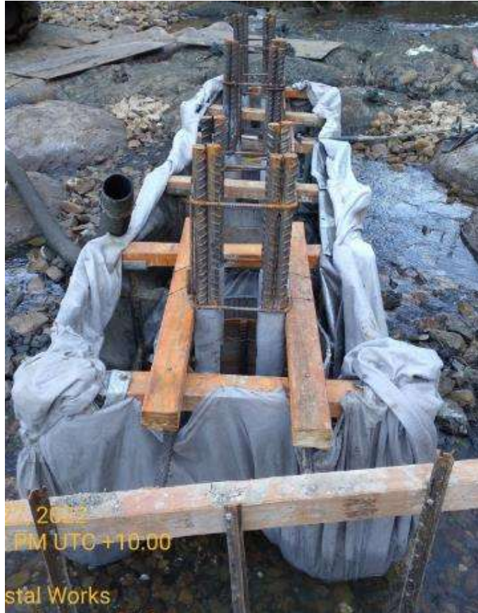
Containment system used for pouring concrete bored piles to prevent concrete overpour entering the waterway
